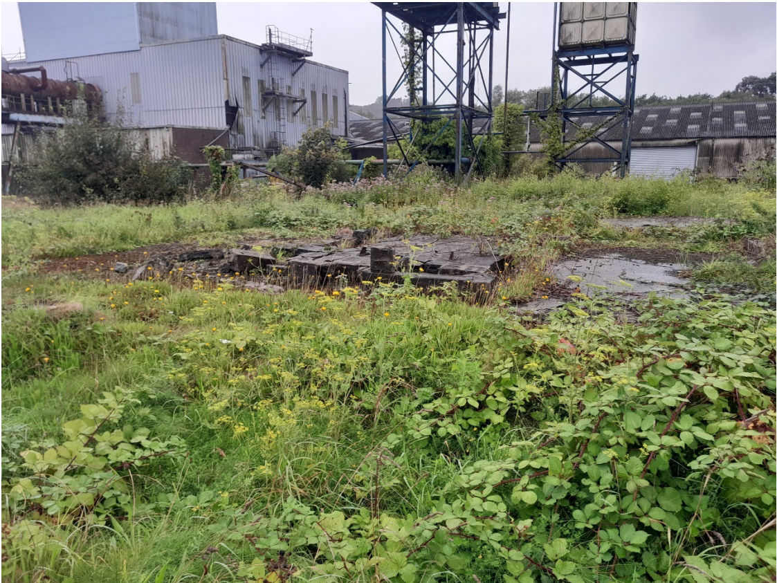
Image EDP A1.15: West facing view of latter 20 th century tank/outbuilding platforms to the east of the Site's building complex.
