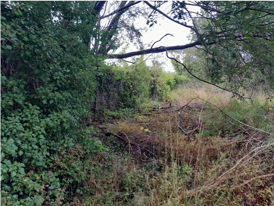
Image EDP A1.24: North facing view of the identified overgrown length of the c. 1901 east stone boundary wall to the Glamorgan Works ( GGAT01225w ). The segment of wall is located to the east of the late 1990s north-south haul road through the Site, hidden by vegetation cover.
