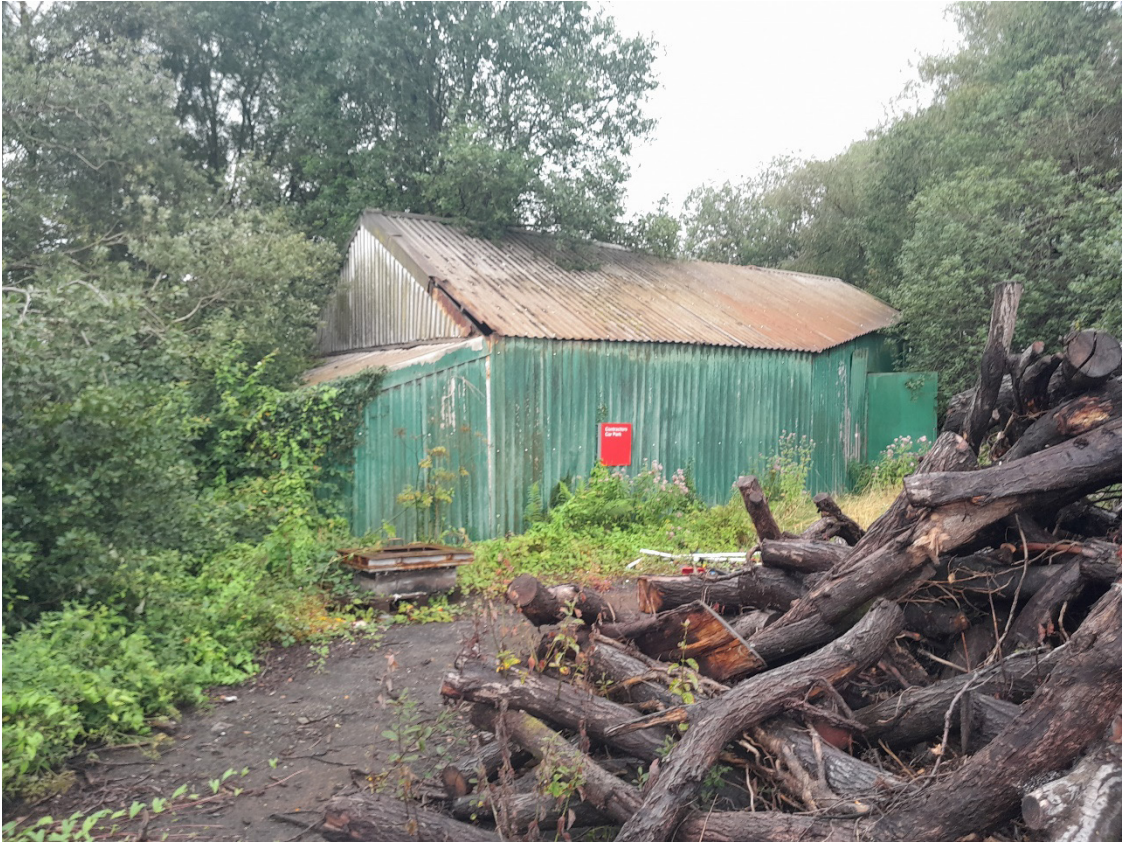
Image EDP A1.6: South facing view of the identified 1960s-1970s corrugated steel shed (1/2) within the south end of the Site.
