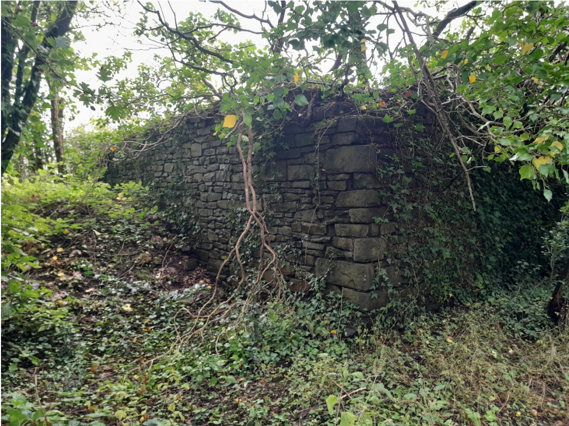
Image EDP A1.23: North-west facing view of the identified overgrown corner of the c. 1901 east stone boundary wall to the Glamorgan Works ( GGAT01225w ). The segment of wall is located to the east of the late 1990s north-south haul road through the Site, hidden by vegetation cover.
