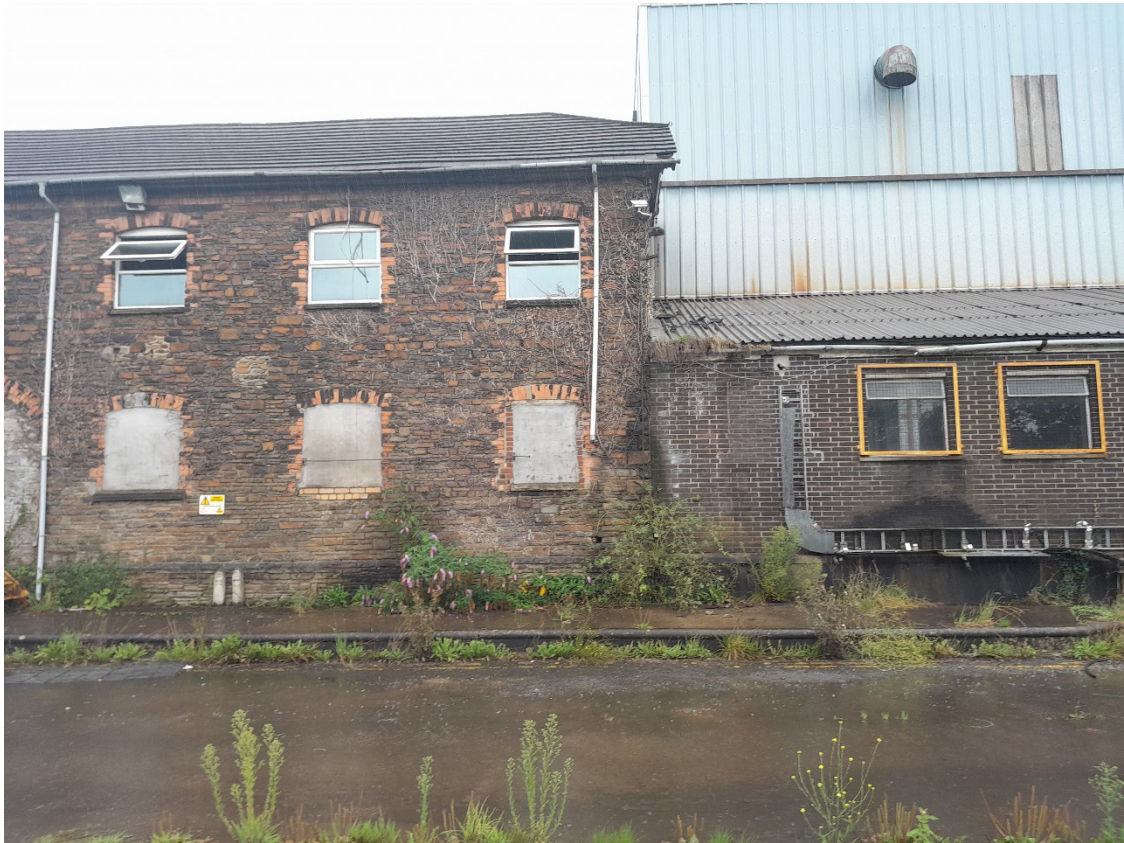
Image EDP A1.12: West facing view of the identified north-south orientated 1870s historic stone-built building (left) and adjoining modern 1972-1992 built post-Glamorgan Works building (right). Modern building is adjoined at edge of building, i.e. dressing quoin stones still present on historic building, showing no sign of the integration of walls.
