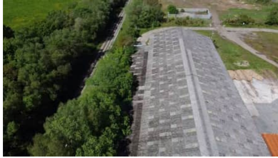
5. Overview of two storey, hipped roofed, stone and brick house (confirmed bat roost).
